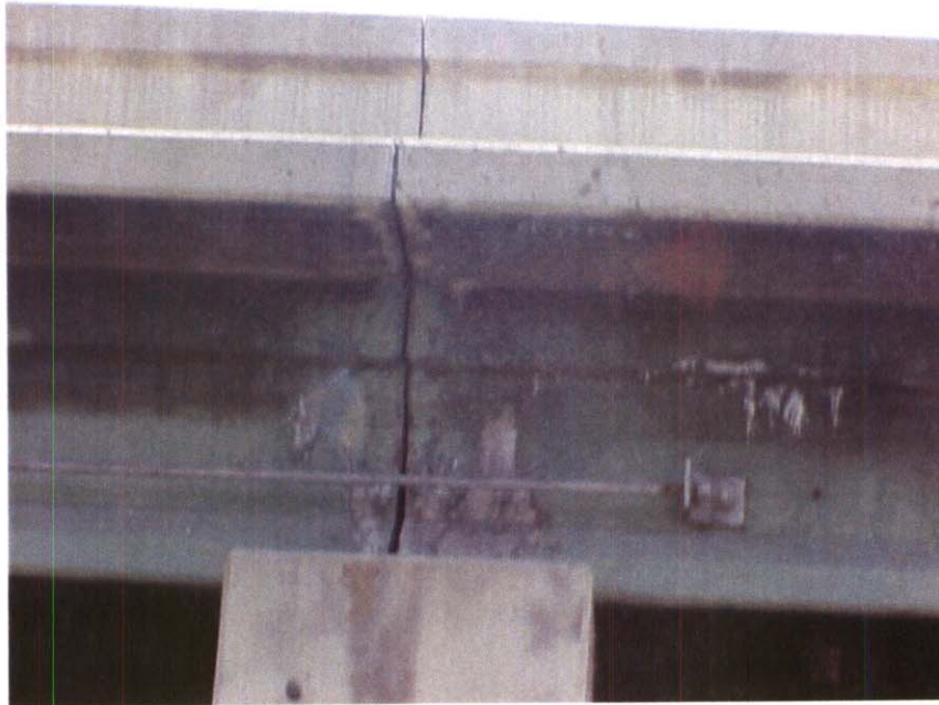
SPANS #1 & #2, CONCRETE "I" BEAMS WITH FINE CRACKS (NOT POOR)
