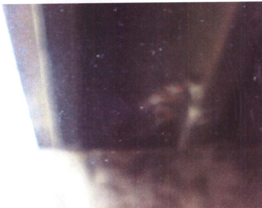
SPAN #2, BOTTOM OF DECK SPALLED TO STEEL
